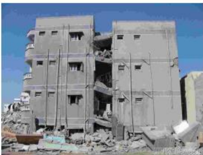
Figure-1. Failure of open first storey in Bhuj Earthquake
